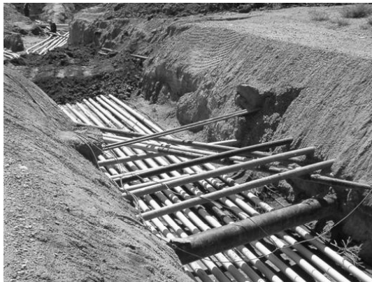
There two types of transmission lines: overhead lines and buried cables.
